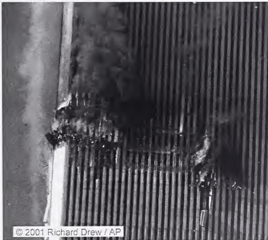
Figure 9-126. Impact Damage to the Northeast Corner of the Exterior Wall of WTC 2.
